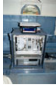
Control electronics and GPS receiver
